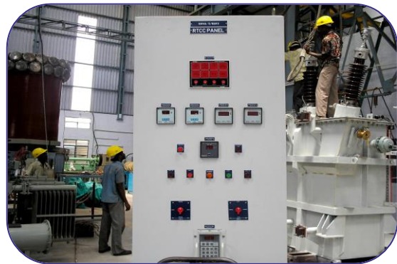
RTCC Panel Assembly
